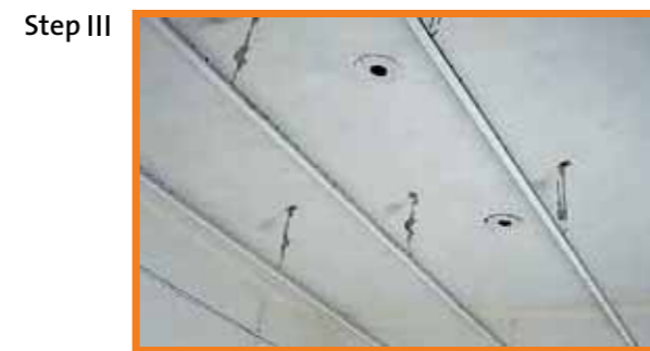
Main "T" sections are suspended from the soffit cleat with the help of level clips
